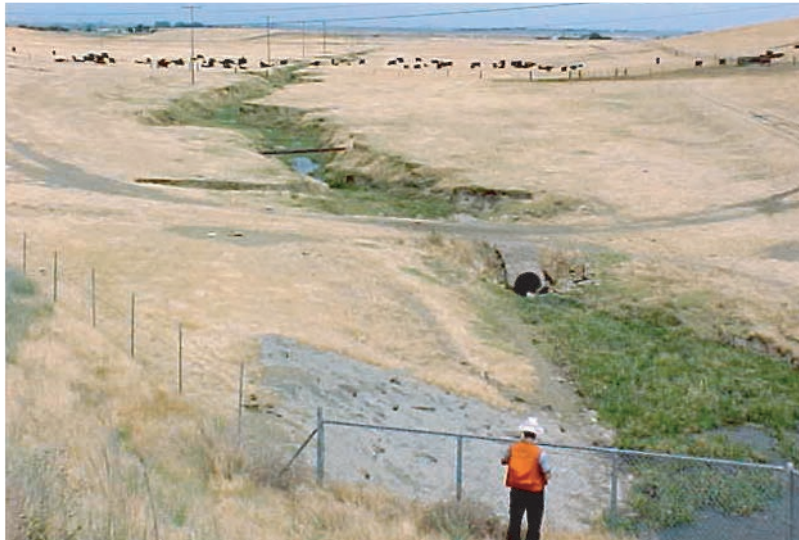
View of erosion caused by cattle and undersized culvert
